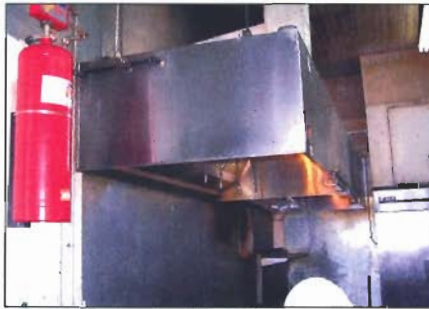
17' Captiveaire Hood & Exhaust System
