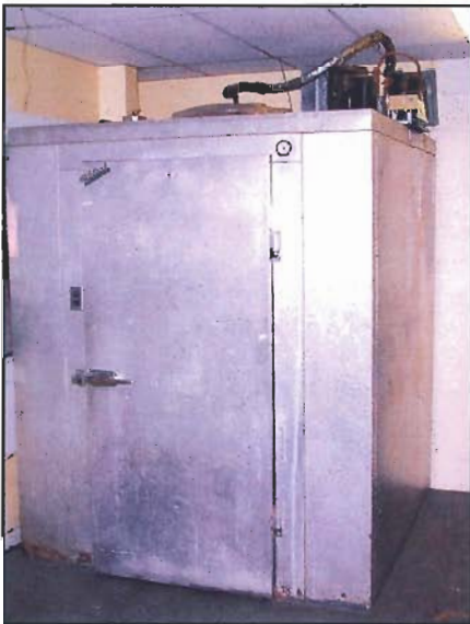
Kolpak Walk-in Cooler
